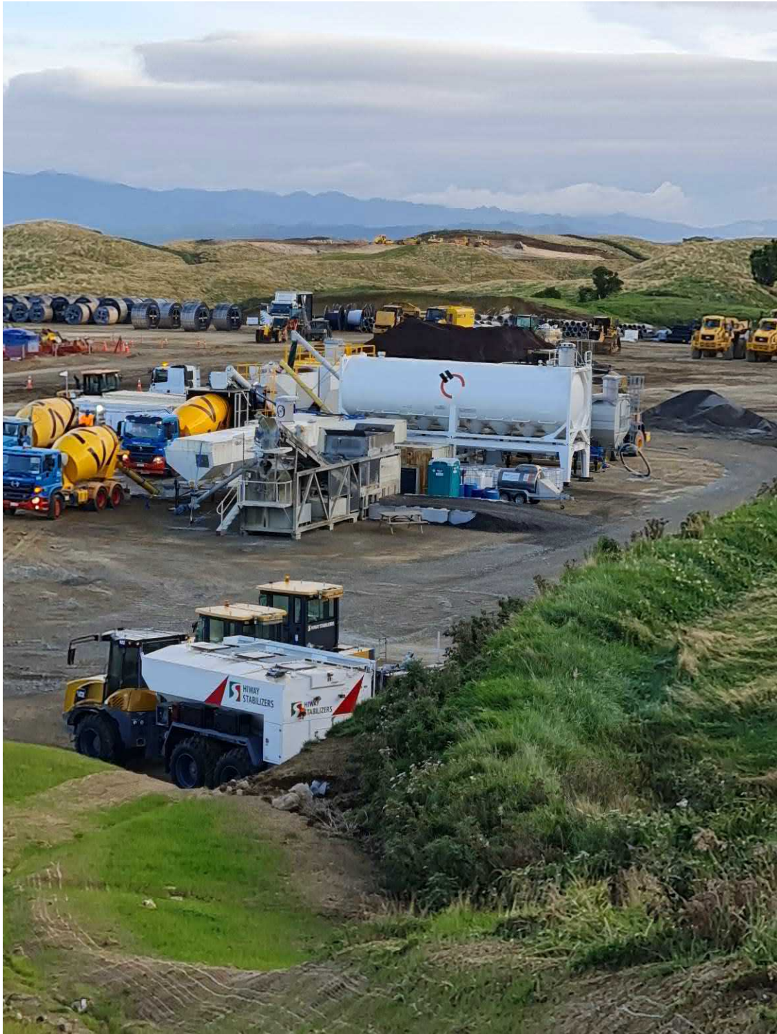
Figure 3: Concrete Batching Plant
